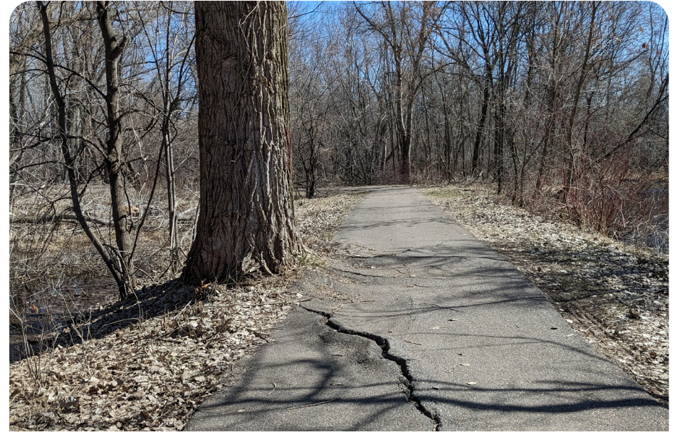
Trees along the trail push up the pavement causing cracks and bumps.
