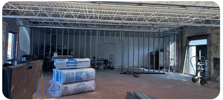
Storage on the north side of the banquet room is framed in.
