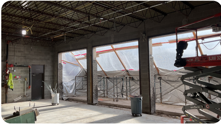
The old garage doors have been removed and it is being prepped for windows.
